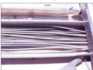
Fire at Mercantile Occupancy, California, April 2009
