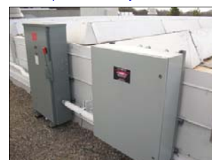
Fire at Educational Occupancy, California, May 2008
