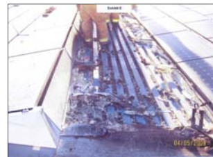
Fire at Mercantile Occupancy, California, April 2009
