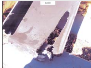
Fire at Mercantile Occupancy, California, April 2009
