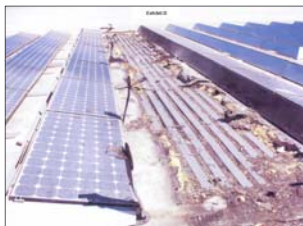
Fire at Mercantile Occupancy, California, April 2009
