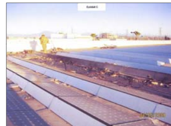
Fire at Mercantile Occupancy, California, April 2009
