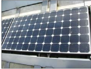
Fire at Educational Occupancy, California, May 2008
