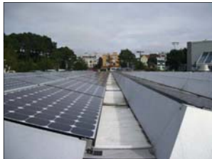
Fire at Educational Occupancy, California, May 2008
