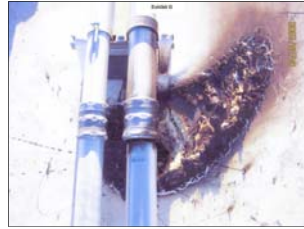
Fire at Mercantile Occupancy, California, April 2009
