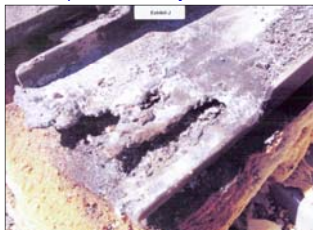
Fire at Mercantile Occupancy, California, April 2009
